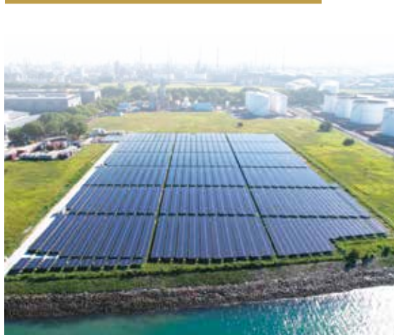
SolarLand panels installed at Jurong Island.
