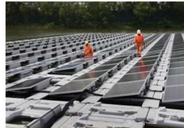
Solar panels at Tengeh Reservoir in Tuas in a photo taken on Oct 21, 2019. PHOTO: The Straits Times
